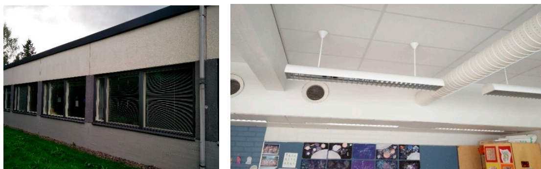
Figure 1. Studied building section, a typical supply air duct diffuser, and an extract air grille in a classroom.
