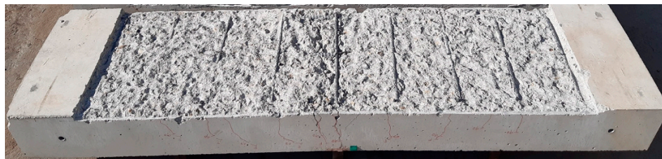
Figure 18. Damaged RC slab after removing strengthened section by chipping.
