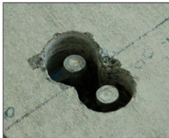
Figure 7. Damage to the connection.
