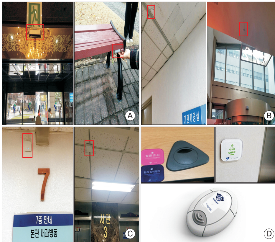
Figure 6. Installation of hardware. (A) Outdoor beacon, (B) indoor beacon, (C) beacon scanner, and (D) NFC tag and wearable beacon.
