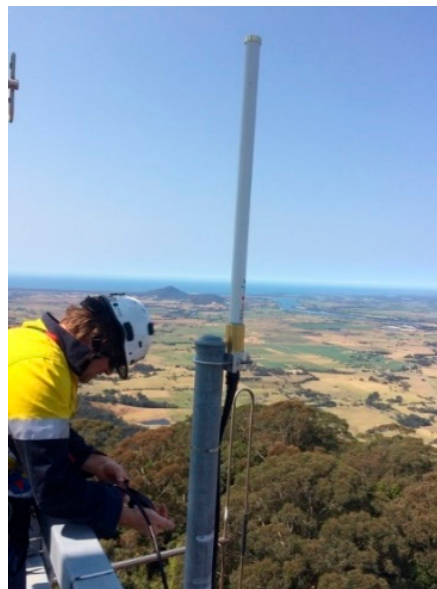
Figure 18. Omnidirectional antenna placement.
