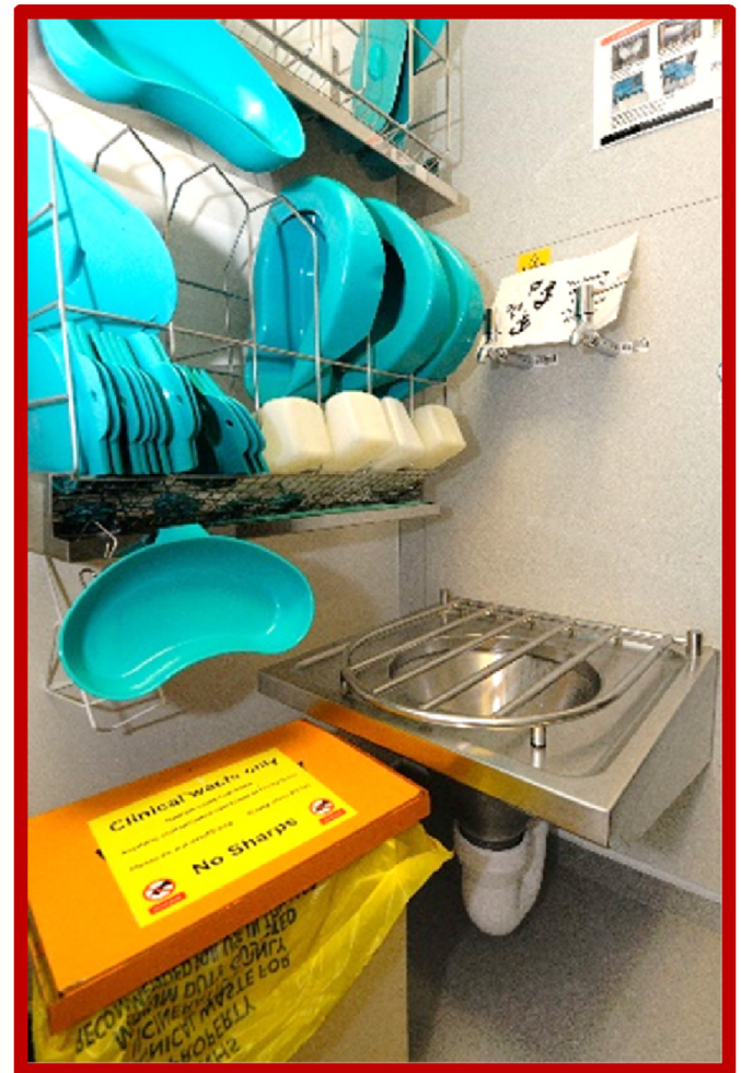
Figure 4. Clean items stored in close vicinity to sluice hopper placing them at risk from splashes/aerosols. Taps above the hopper will cause significant splashing when used.
