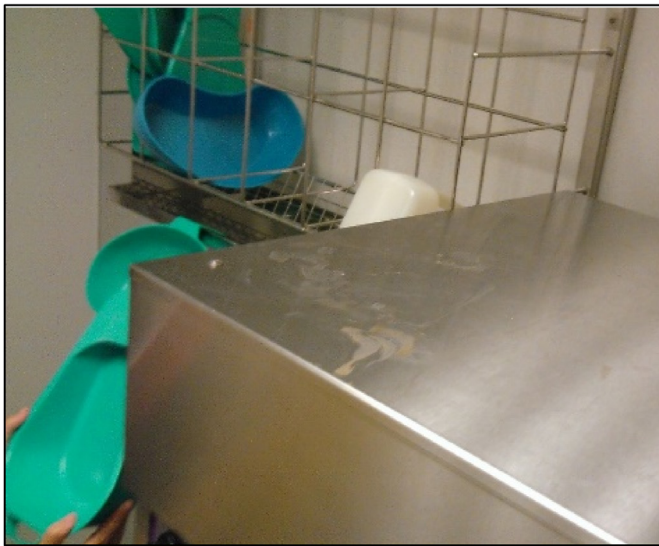
Figure 3. (a) A nurse standing in front of a bedpan washer disinfectator. These items are quite tall making it difficult to see any contamination on the top surface. (b) Faecal contamination of the top surface of the washer disinfectator.
