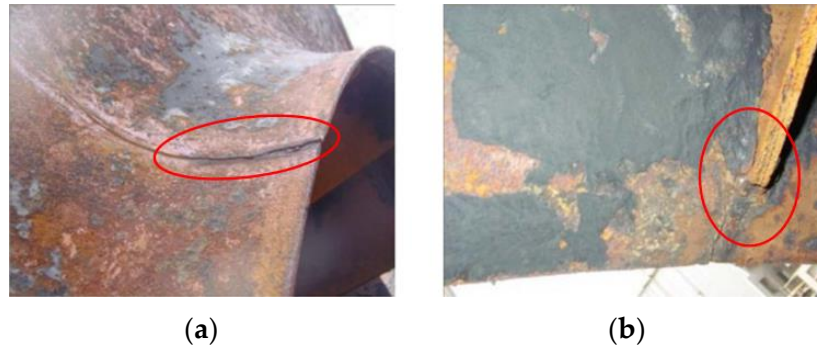
Figure 22. Photo of the crack on B fan.
