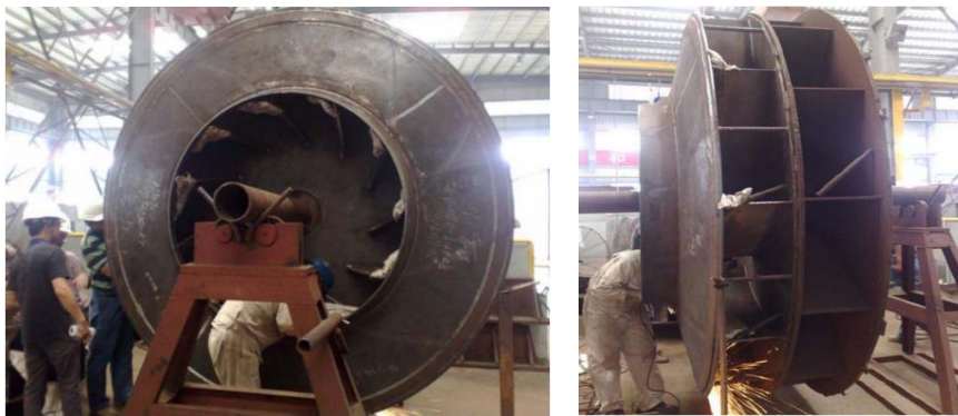
Figure 3. Photos of the rotor blades of No. A fan.
