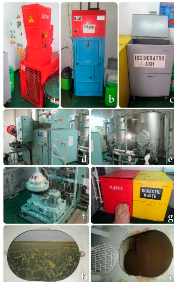
Figure 3. (a) Units involved in waste management on board ships: ship waste shredder; (b) ship waste compactor; (c,g) ship-generated waste collection and segregation; (d) ship waste incinerator; (e) oil derivatives processing tank; (f) oil separator unit; (h,i) oily bilge water and bilge well. Photo: Paweł Borowski.
