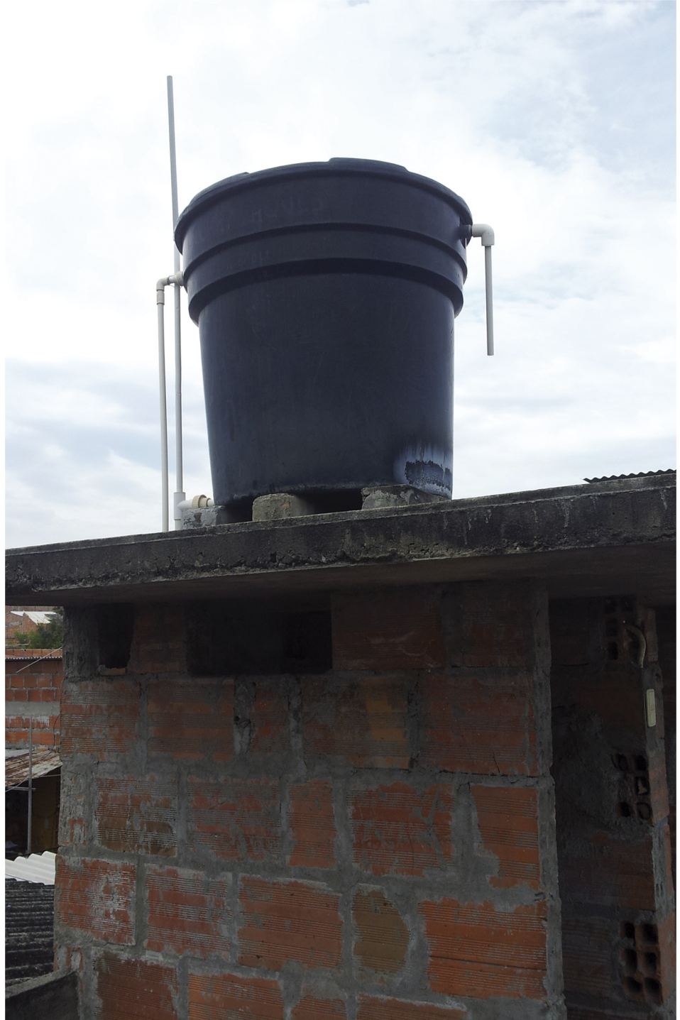
Fig 2. Tank: Cylindrical structure made of plastic or fiber cement with a capacity superior to 250 liters.
