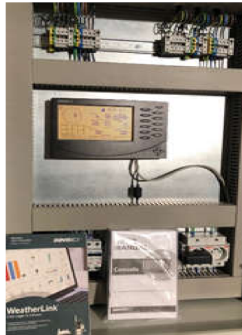
Figure 11. Installation monitoring and verifying the environmental parameters of the performance of a modernized ribbon-blade wind turbine. The installation verifying the environmental parameters of the modernized ribbon wind turbine is the end of the telecommunication sewage system monitoring (point 3—Figure 8). Source: the authors' own materials (based on R. Kasner).
