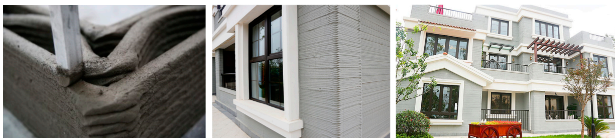
Figure 18. A 3D-printed three-story villa by Winsun in Wujiang, China. Figures reproduced with permission from [198].
