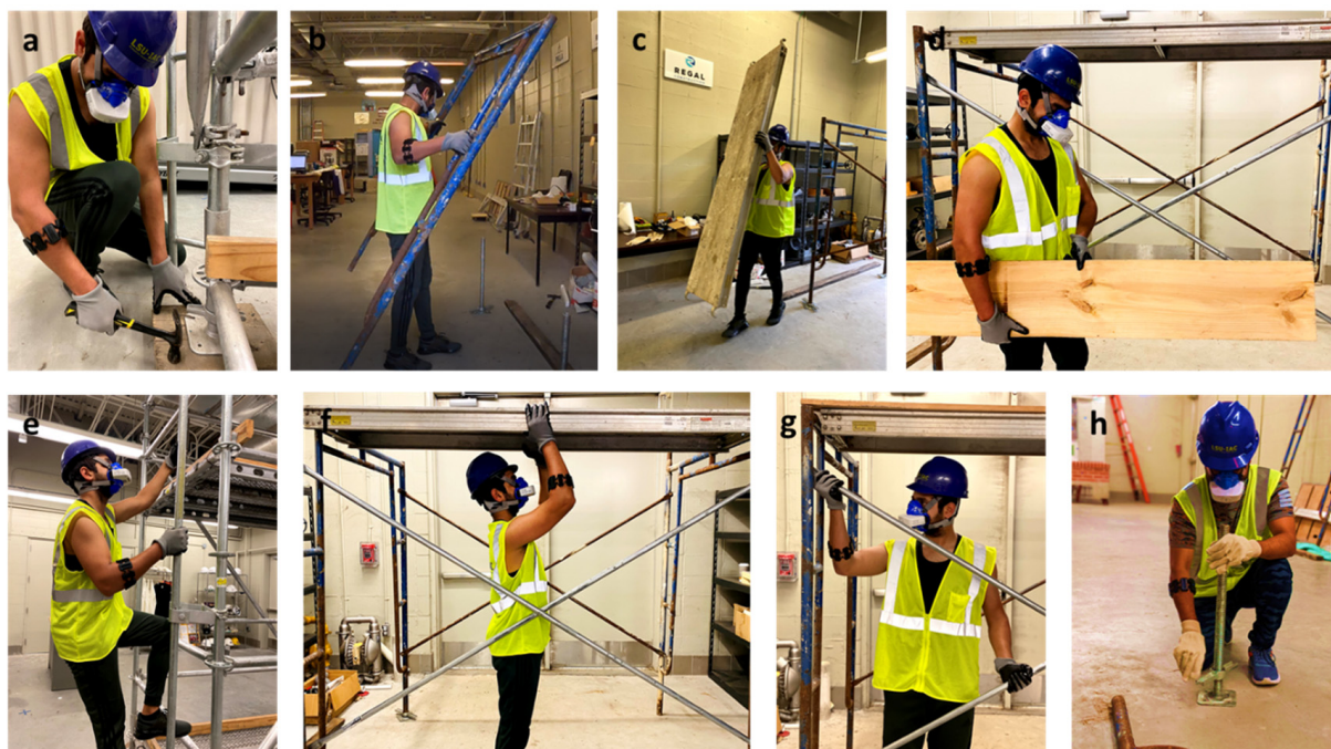
Figure 1. Participants performed different scaffold-building activities. (a) Hammering, (b) carrying scaffold frame, (c) carrying baseboard, (d) carrying guardrail, (e) going up the vertical ladder, (f) installing baseboard on a different level, (g) installing crossbars, and (h) adjusting leveling jacks.
