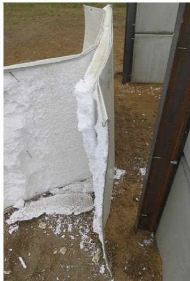
Figure 13. Displacement of the sandwich panel from the supporting structure.
