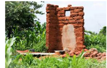
Poor sanitation infrastructure
