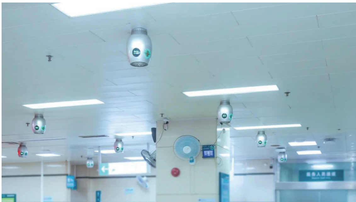
FIGURE 1. Ceiling oxygen equipment in the outpatient hall.
