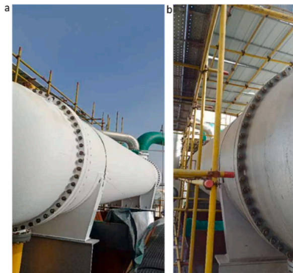
Fig. 3. Photographs of carbon steel-based chemical pipelines with (a) and without (b) the SSC-HE coating.
