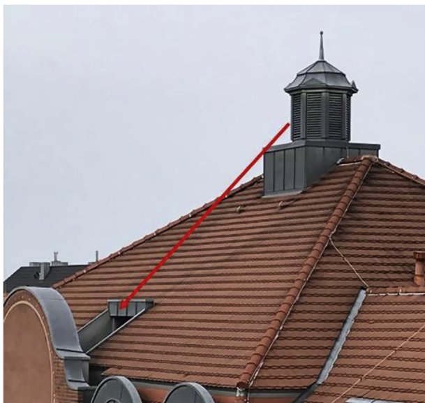
Figure 4. Exhaust air opening in the tower at the highest point of the roof building of the nursing home as well as the location of the supply air opening (red arrow).
