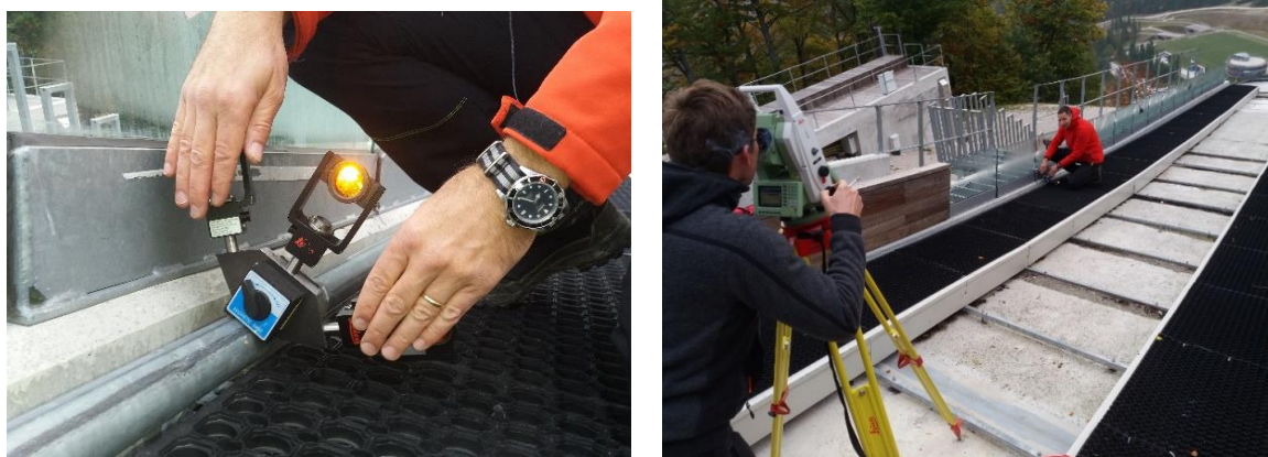
Figure 11. Measurements with the multi-prism method and the covering of two prisms during measurements on the inrun of Planica ski-flying hill.
