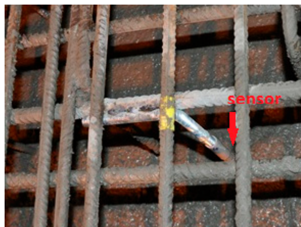
Figure 2. Photograph of an ultrasonic transducer mounted at a bridge construction site before casting (Photo: Neostain S.A.).
