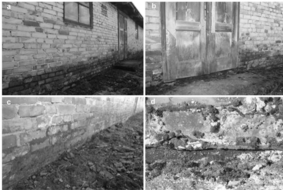
Figure 3. Biodeterioration symptoms of external part of buildings (numerical value of deterioration in a 4-point scale). a) capillary rise of groundwater; area adjacent to the building covered by concrete rubble mixed with soil (3– intensive changes); b) door colonized by algae and cyanobacteria, mosses and lichens on the ground (2– moderate changes); c) concrete rubble mixed with soil, colonization by algae and mosses (3– intensive changes); d) colonization by lichens and mosses, horizontal moisture insulation damaged (3– intensive changes). doi:10.1371/journal.pone.0109402.g003
