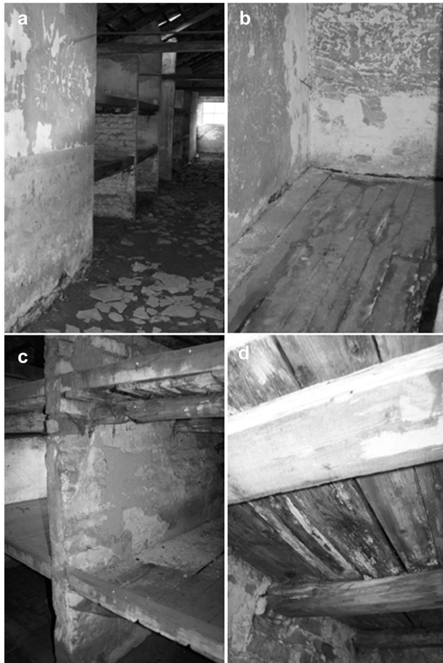
Figure 4. Biodeterioration symptoms of internal part of buildings (numerical value of deterioration in a 4-point scale). a) the middle part of building, damages of the floor (3– ground floor: intensive changes, 2– walls: moderate changes); b) block master’s room and storeroom, damages of the wood floor, algae and cyanobacteria colonization (3– ground floor: intensive changes, 1– walls: small changes); c) bunk bed partitions, bulging and crumbling plaster (3– intensive changes); d) damages of bunk beds board caused by wood-decaying fungi (2– moderate changes, locally).
