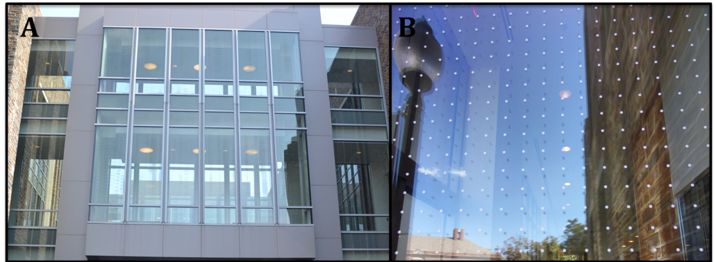
Figure 5 Bird deterrence dotted patterns on windows of Fitzpatrick building at Duke University. (A) Glass passageways. (B) Close up of dotted pattern. Photos: Casey Collins.
