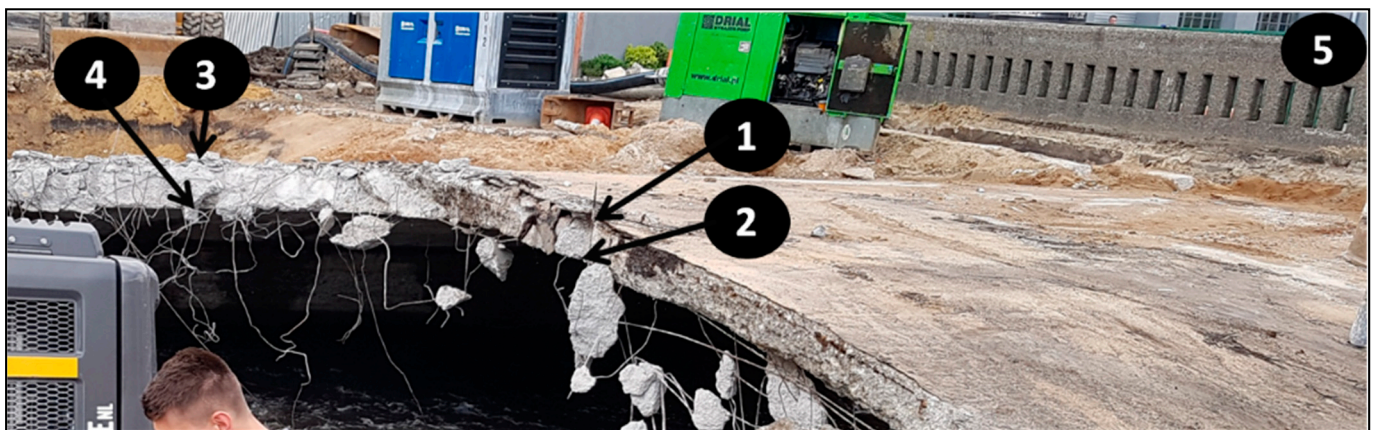
Figure 6. The RC (reinforced concrete) slab after removing the bituminous layer from the bridge.
