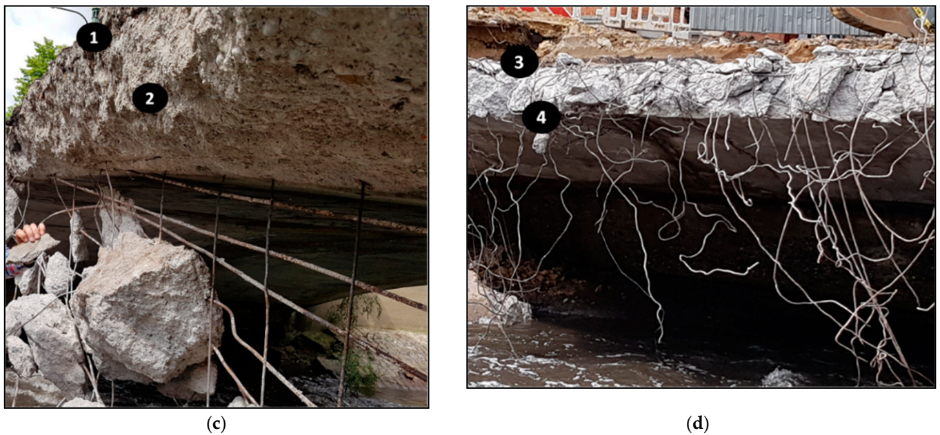
Figure 5. The sampling sites during demolition: Corroded steel mesh and carbonate icicles: (a) location of samples 2 and 4, (b) location of samples 2, (c) location of samples 1 and 2, (d) location of samples 3 and 4.
