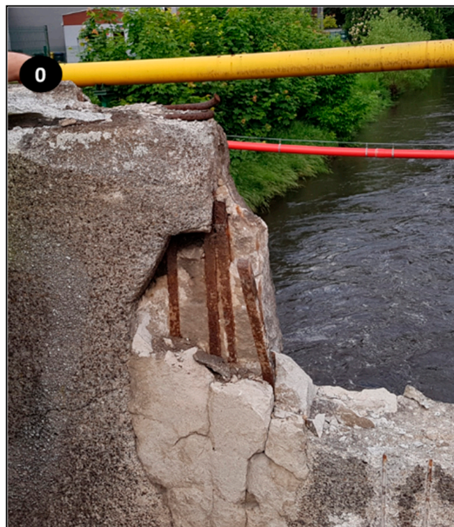
Figure 8. Corroded steel bars in the concrete of the balustrade.
