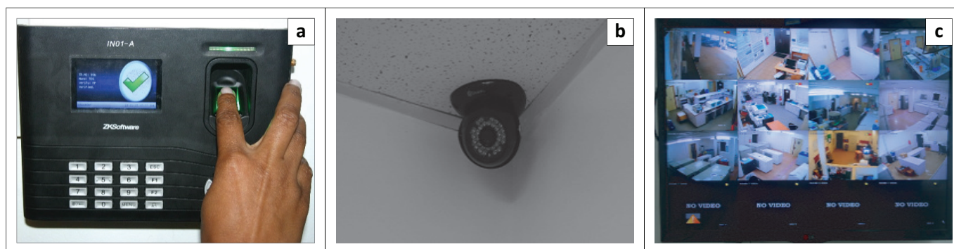
FIGURE 5: Security installations at Institute of Human Virology Nigeria H3Africa biorepository. (a) Biometric access control panel. (b) Motion-activated closed circuit television camera. (c) Monitor display from closed circuit television camera showing both interior and exterior areas of biorepository.
