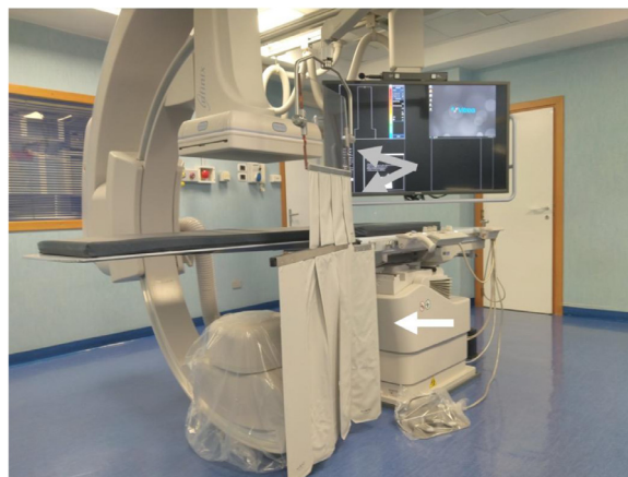
Figure 6 Angiosuite with leaded x-ray protections (white arrow: low protection with leaded curtain; gray arrows: high protection with leaded curtain and leaded glass).
