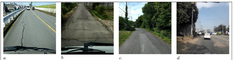
Fig. 5. Sample images for road damage categories considered in the data. a. Longitudinal Crack (D00) b. Transverse Crack (D10) c. Alligator Crack (D20) d. Pothole (D40).
