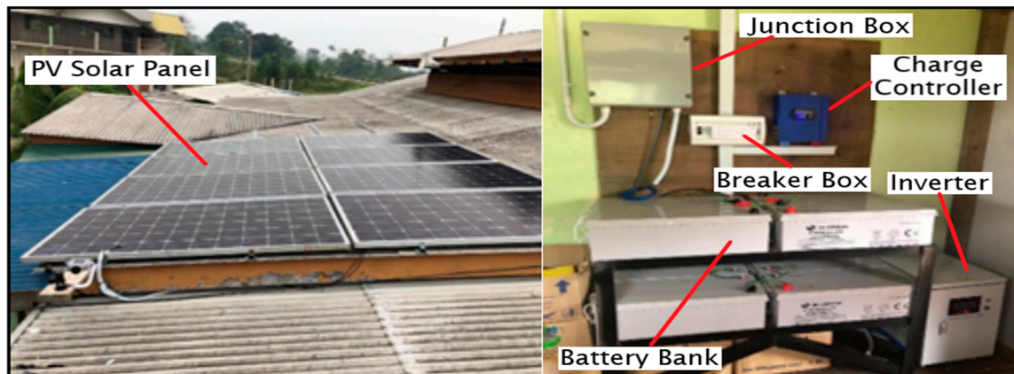
Figure 2. Installation of stand-alone solar system.
