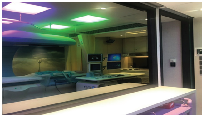
Figure 4: The appearance and colored lighting of the high-intensity focused ultrasound operating theater
