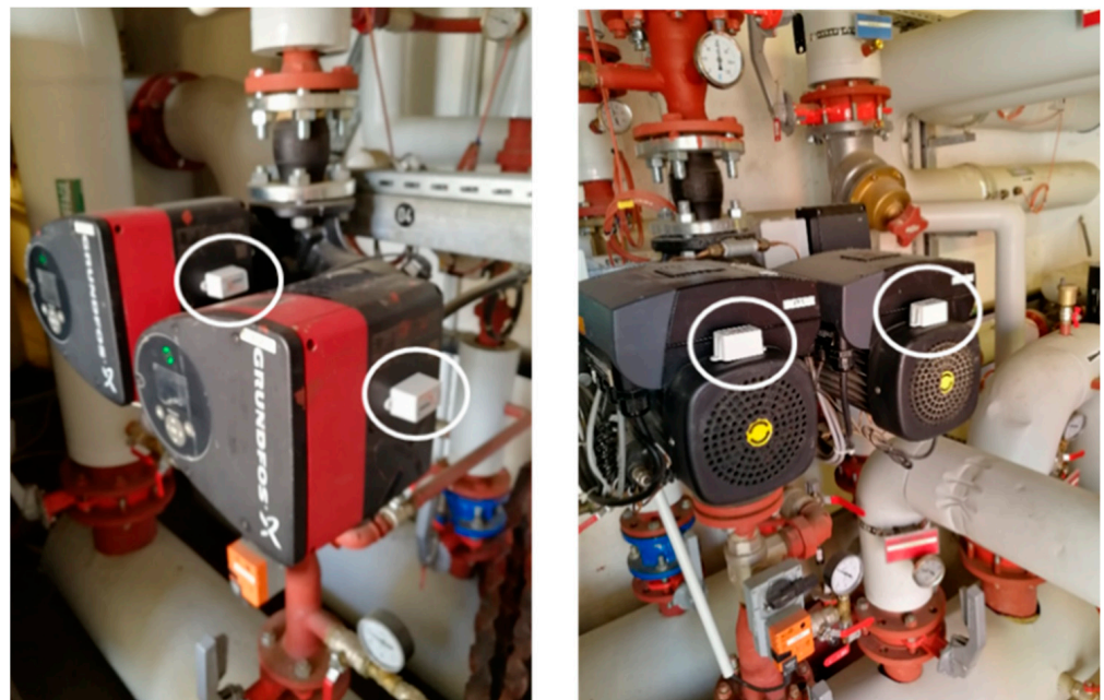
Figure 5. A photo of a vibration device installed on a double pump.
