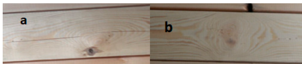
Figure 7. The appearance of critical areas of lumber forming the face of the P34 beam—exterior side of the beam.
