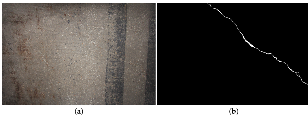
Figure 8. (a) Sample crack image and (b) annotated image from the Illinois Bridge dataset.
