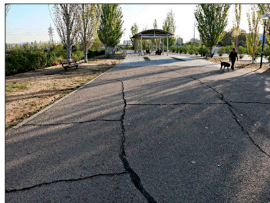
Photograph: “Broken ride”
