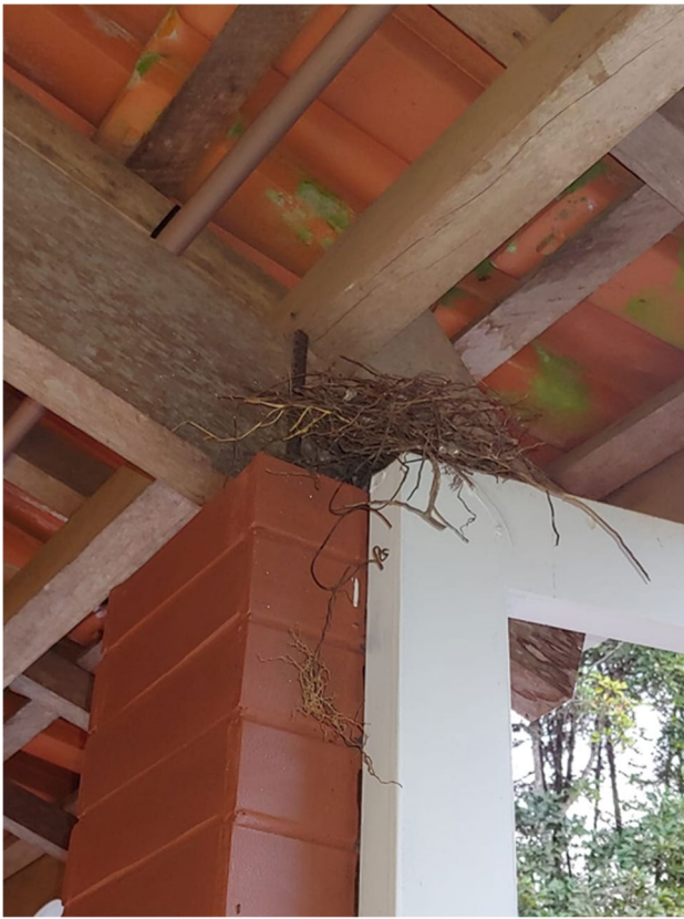
Fig. 5 Abandoned nest built in the house roof lining
