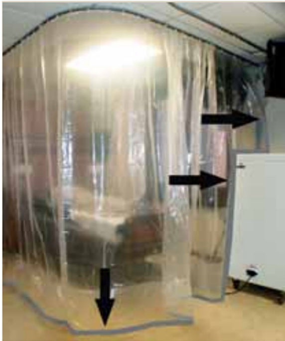
Figure 6. Temporary negative pressure isolation: like a clinical construction set-up, a plastic curtain is connected to ceiling and wall with a zippered entry, and an in-circuit HEPA filtration system for one-pass air. Reproduced from public reference (7). HEPA, high-efficiency particulate air. (Color version of figure is available online.)
