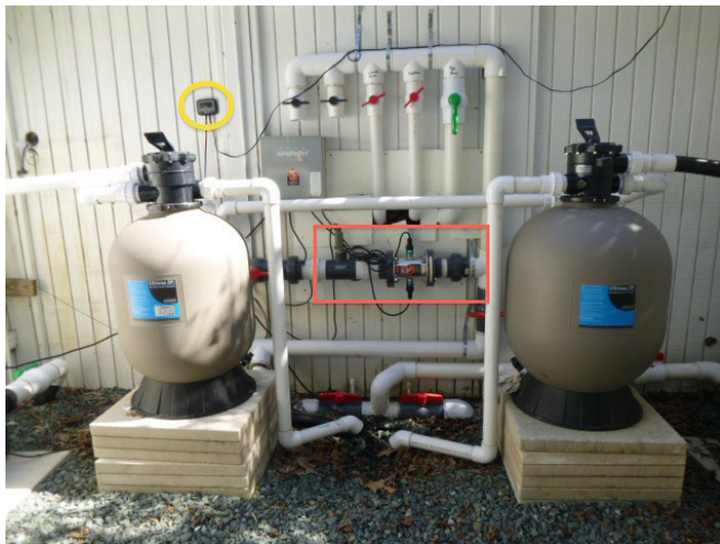
Figure 1 Life support system for backyard pond. Two 400W UV filters are shown in the red rectangle. IonGen copper ion generator is shown in the yellow circle. The life support system also contained two pumps and advanced biological filtration.
