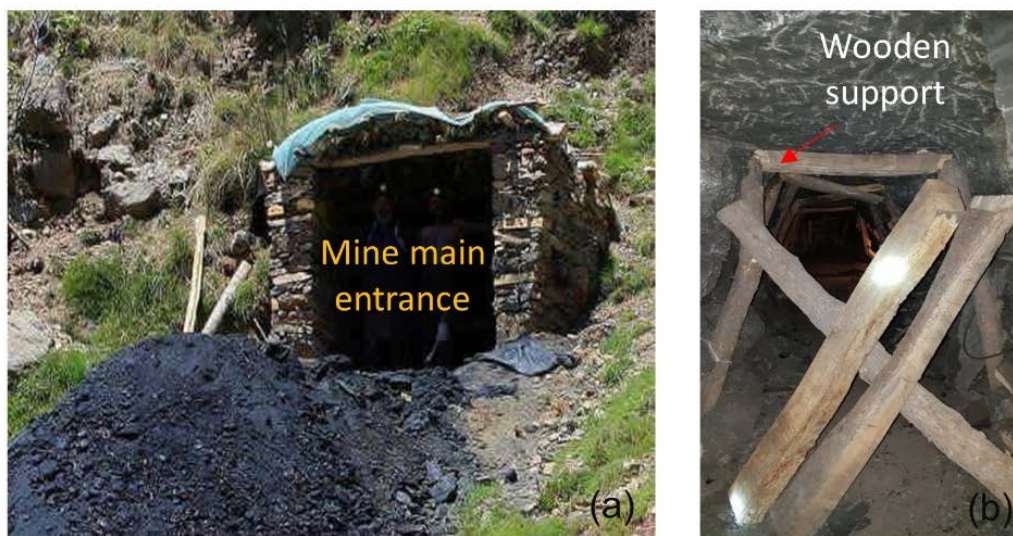
Figure 7. (a) Mine portal opening, (b) a closed entry of the mine with installed wooden support.
