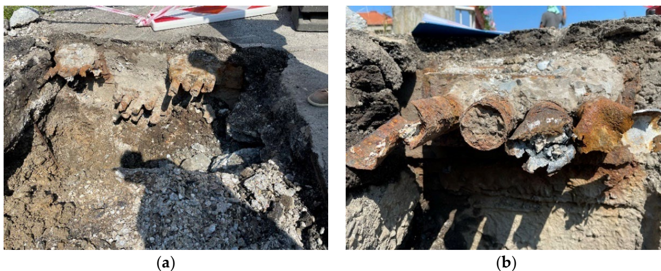
Figure 8. Anchorage area at the end of the beam—view (a); detail (b).
