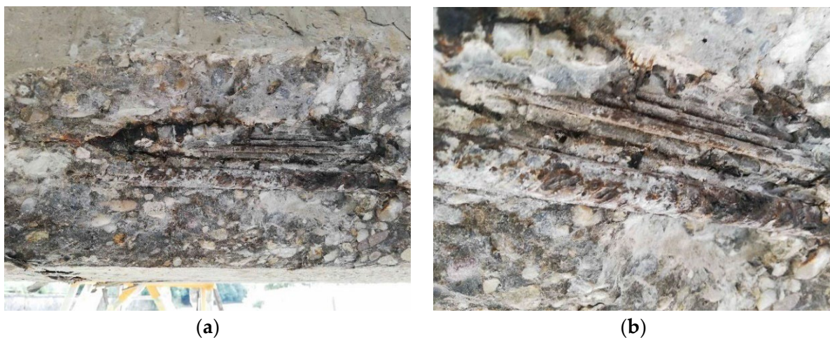
Figure 5. Prestressing wires after exposure in the midspan area—view (a); detail (b).
