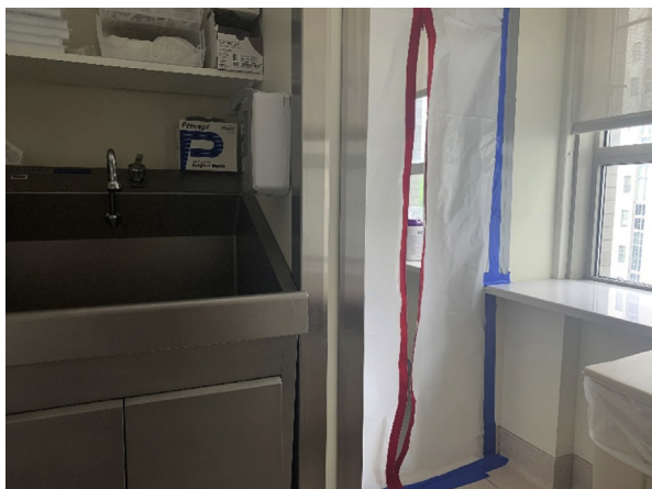
Figure 2. A hallway connecting the procedure room and control room was converted into an anteroom through the use of floor-to-ceiling plastic barriers with zippers.
