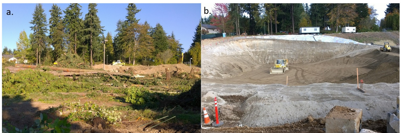
Fig 1. Commercial development project located in Redmond, Washington. Depicted: a. clearing the site of vegetation and b. grading the site and digging the foundation. Photo credit: K. Dyson.
