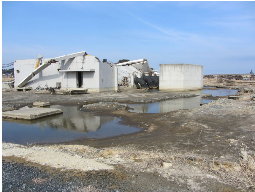
Figure 1. A scene following the 2011 Heisei Tsunami in Idagawa, Fukushima, Japan, showing destruction of a reinforced-concrete structure and severe scour surrounding the structure.
