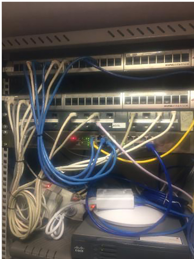
FIGURE 3 'The wires are a mess part two' by P1.
