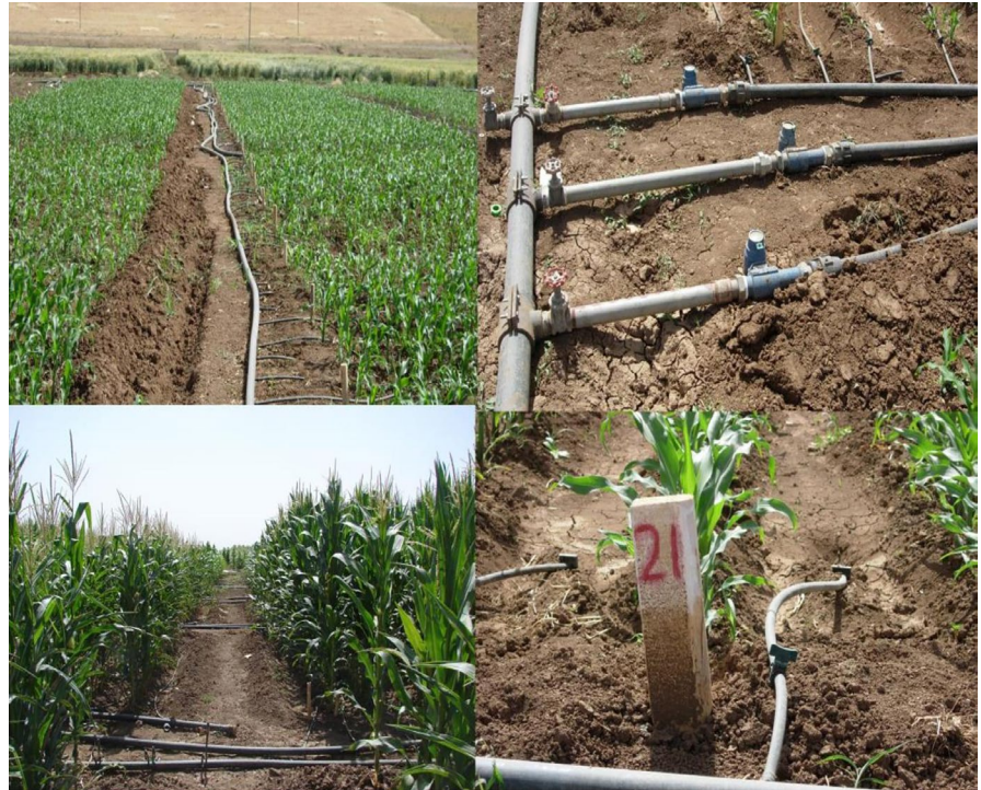
FIGURE 2 Irrigation system and controlling the amount of water required
