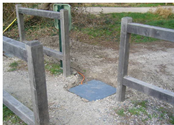
Figure 7. Eco Counter ‘SLAB’ installed at a pedestrian pinch point.
