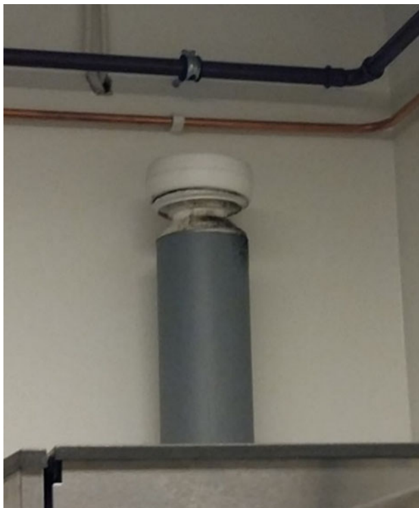
Fig. 2. The implicated white coloured air ventilation valve and its grey connecting ventilation sink behind the ice cube machine.
