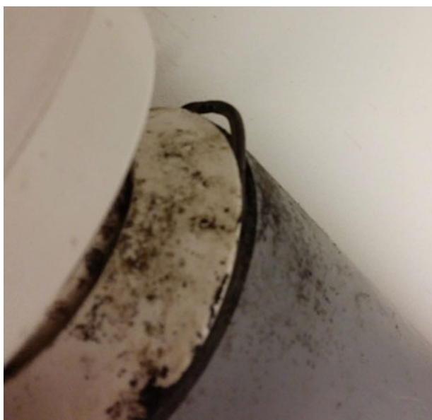
Fig. 3. Black smudge on the right-hand side on the neck of the valve where the valve was leaking.
