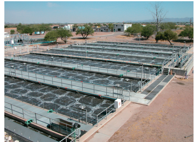
FIGURE 24.8 Secondary treatment: an aeration basin. From Pepper, Gerba, and Brusseau, 2006.
