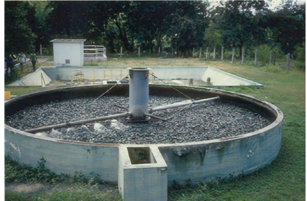
FIGURE 24.7 A trickling filter bed. Here, rocks provide a matrix supporting the growth of a microbial biofilm that actively degrades the organic material in the wastewater under aerobic conditions. Photo C.P. Gerba.
