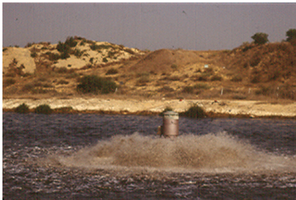
FIGURE 24.16 An aerated lagoon.
