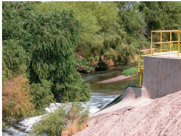
FIGURE 24.20 Effluent outfall of the Roger Road Wastewater Treatment Plant in Tucson, Arizona. Here, extensive growth of vegetation due to the effluent produces a riparian habitat. From Pepper, Gerba, and Brusseau, 2006.
