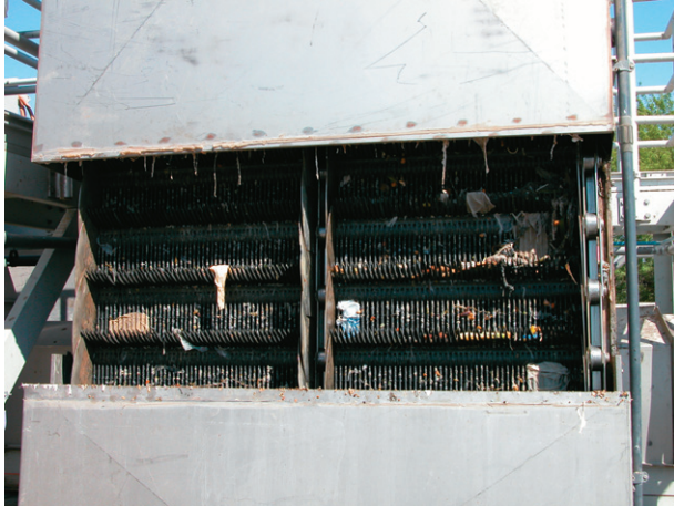
FIGURE 24.4 Removal of large debris from sewage via a bar screen. From Pepper, Gerba, and Brusseau, 2006.
