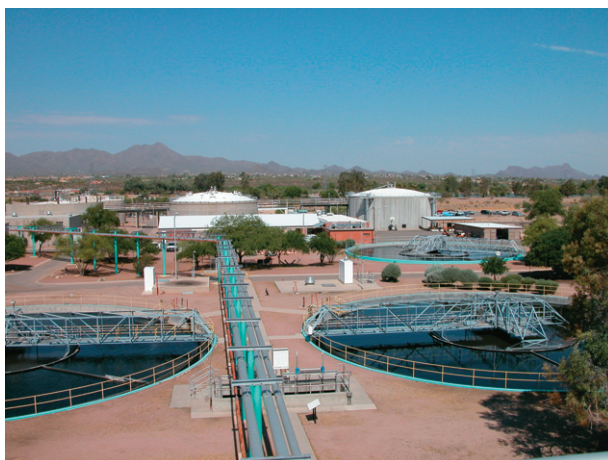
FIGURE 24.6 Three clarifiers (foreground—blue) where suspended organic solids settle out as primary sludge. Also see the two anaerobic sludge digesters in the background (white). From Pepper, Gerba, and Brusseau, 2006.
