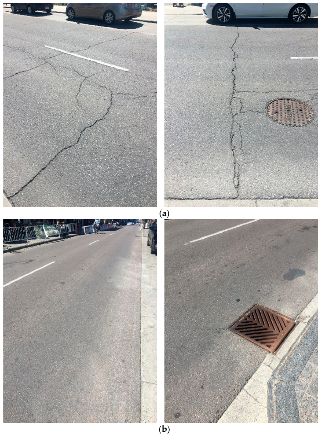
Figure 1. (a) Representative photographs of pavement reconstructed in 2010 on three blocks of Princess Street and King Street in downtown Kingston, Ontario, (b) Representative photographs of pavement reconstructed in 2011–2012 on seven adjacent blocks of Princess Street.
