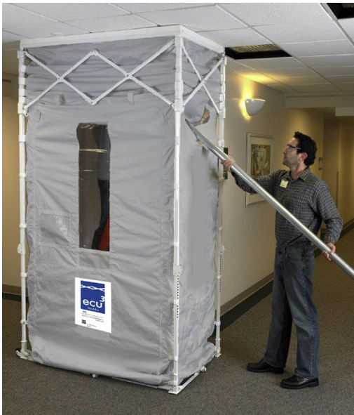
Fig. 8. Portable containment device for above-ceiling work. (From Olmsted RN. Prevention by Design: Construction and Renovation of Health Care Facilities for Patient Safety and Infection Prevention. Infect Dis Clin North Am. 2016 Sep;30(3):713-28; with permission.)
