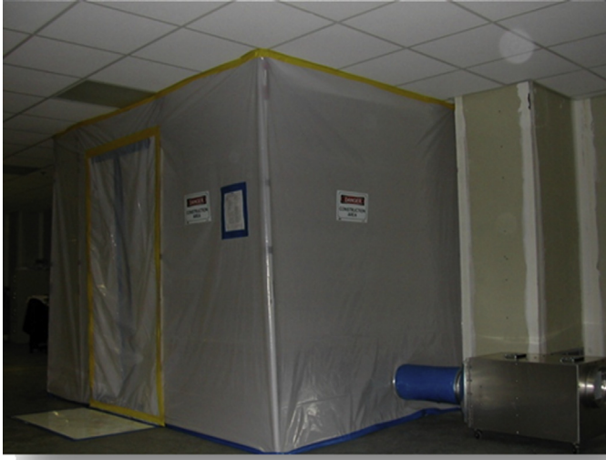
Fig. 9. Barrier separation and containment of active construction zone from occupied areas. (From Olmsted RN. Prevention by Design: Construction and Renovation of Health Care Facilities for Patient Safety and Infection Prevention. Infect Dis Clin North Am. 2016 Sep;30(3):713-28; with permission.)
