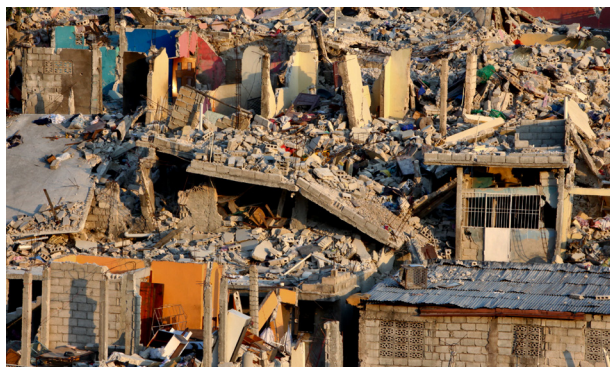
Figure 5. Closer view reveals the crumbling of masonry construction and weak column joints. Note no collapse of nonengineered building with light aluminum roofing on the right.
