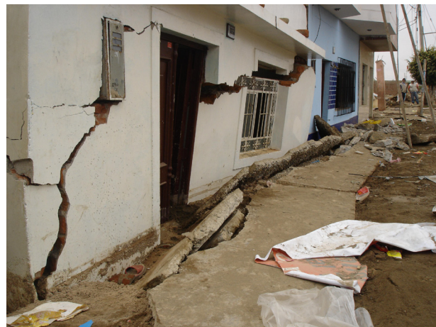
Figure 6. The situation was better in Peru where reinforced concrete was used. However note that 45 degree earthquake cracks from shear forces can be seen on masonry structures.
