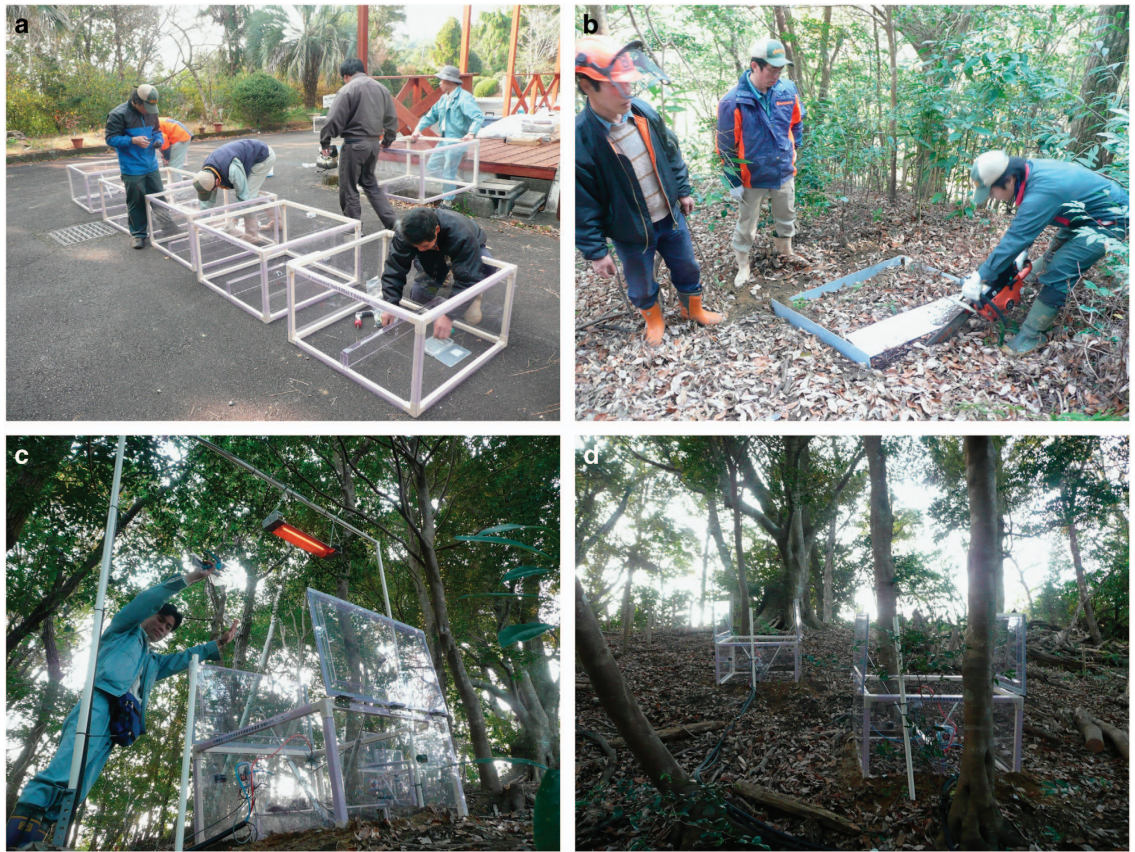
Figure 3. Chamber system installation at the Miyazaki Experimental Warming Site. (a) The chambers were assembled in the field. (b) Trenches were created using a chainsaw to sever roots. (c) The carbon-filament heat lamp was installed above the warming chamber. (d) Photograph of the study site with the chambers installed. The authors affirm that the individuals depicted herein provided informed consent for the use of their images.
