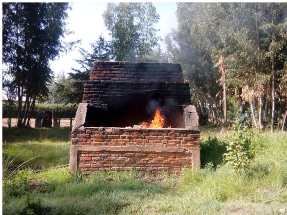
Fig. 1 Poor condition of a brick incinerator at Bale zone hospitals, Southeast Ethiopia, 2018
