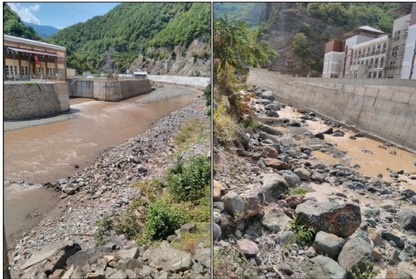
Fig. 14. The common application of constructing concrete walls along the streambed to stabilize the banks to protect both the roads and RoR-HEPP facilities (on the left), and houses/buildings (on the right) in the lower part of the Murgul Stream.
